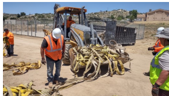
Staff was able to use the Public Works department's heavy equipment to load bulky items into dumpsters
